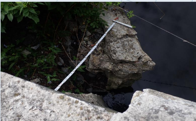
SE wingwall broken free from the culvert (Top View)
