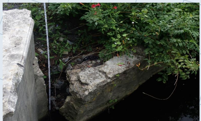
SE wingwall broken free from the culvert (Front View)
